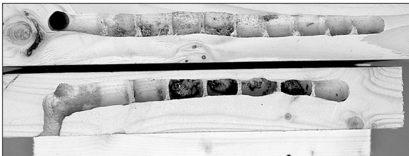
Wood damage caused by carpenter bee gallery construction.
